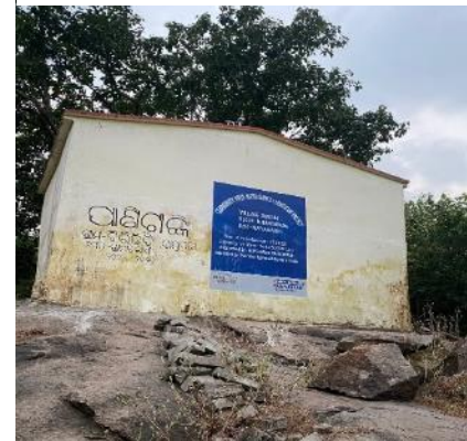
Image 4: Overhead water tank
